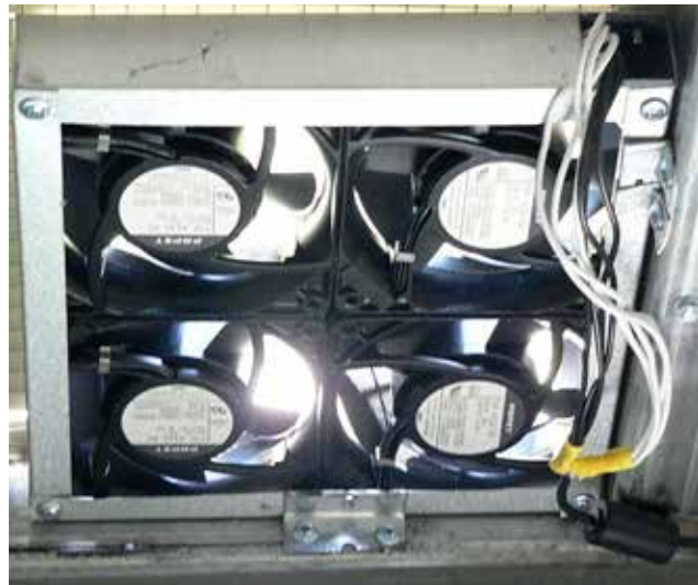
EXHAUST FANS AT FLOOR LEVEL
